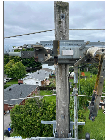
(b) Overhead switch operational defect
