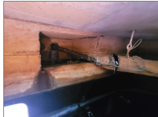
(b) Underground cable failure
