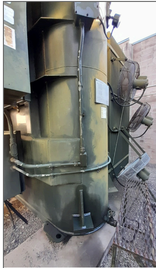
(a) Station transformer corrosion and leaks
