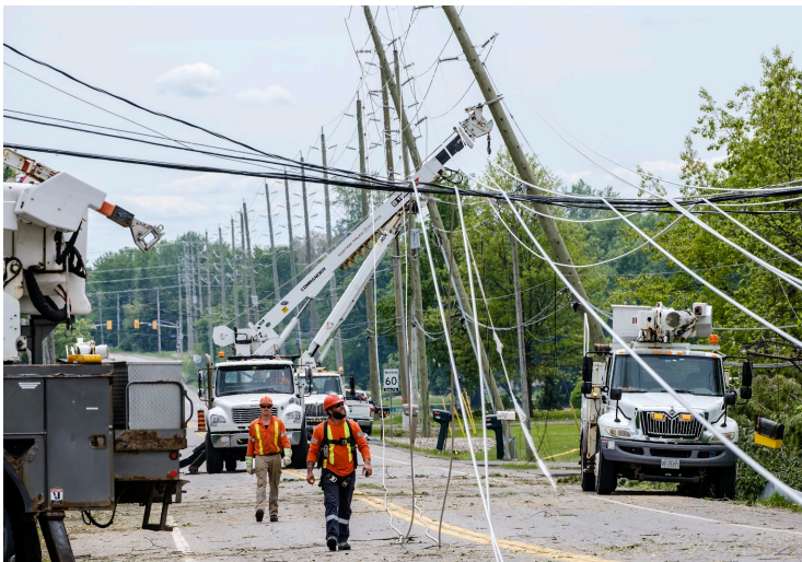
Assessing Damage after the 2022 Derecho
