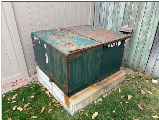
(a) Underground transformer corrosion
