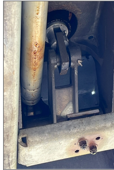
(b) Switching equipment lubrication leaks
