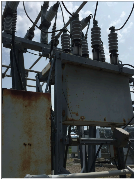
(e) Station outdoor infrastructure deterioration
