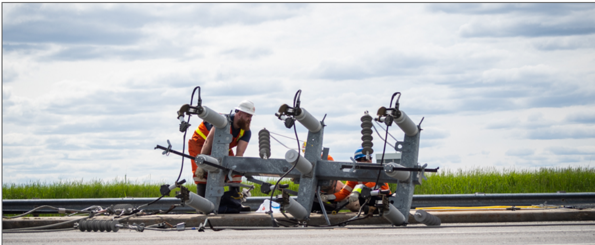
Clearing damaged equipment after the May 2022 Derecho
